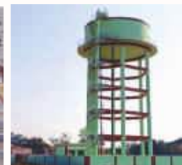
Over Head Reservoir
